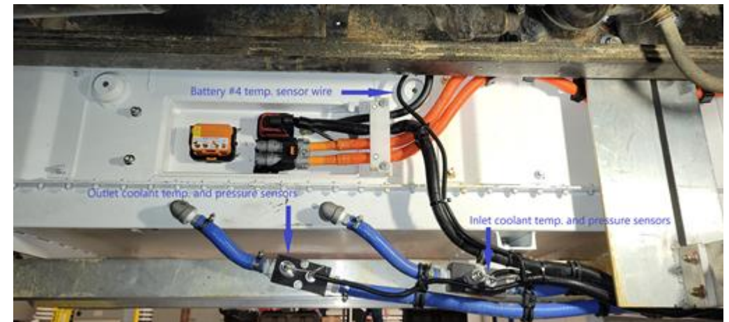
Battery pack instrumentation for thermal evaluation
