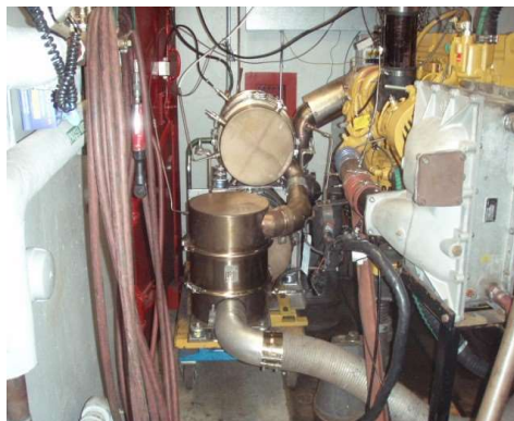
Figure 1 - Diesel-Particulate-Filter Low NO 2 -CRT emission control device and Caterpillar C 11 diesel engine installed in the CANMET test cell
