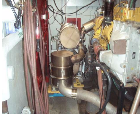
Figure 1 - Diesel-Particulate-Filter Low NO 2 -CRT emission control device and Caterpillar C11 diesel engine installed in the CanmetMINING test cell
